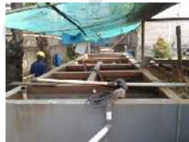
CLEAN WATER POND
